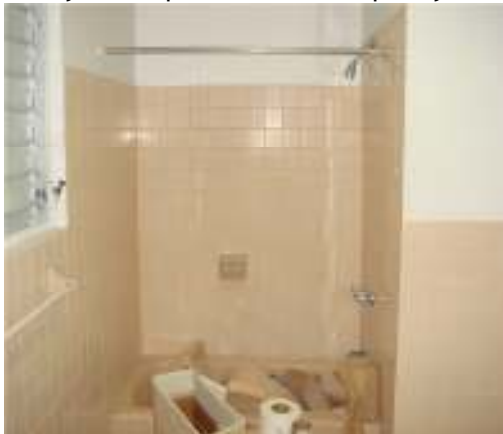
Old Obsolete Restroom
